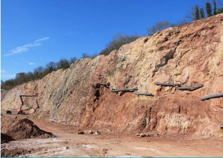
The installation site was suffering from severe surface erosion
