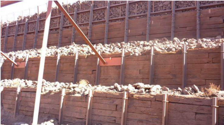
The Terraced North Wall Showing Signs Of Distress
